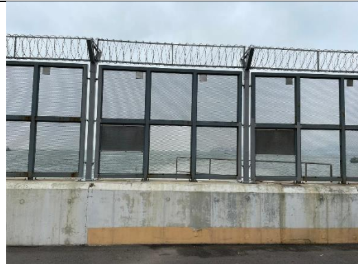
Cooling Water Discharge Facility for CCGT Unit No.1 and reinstatement of crest walls and fencing barrier
