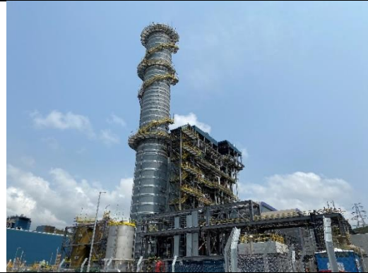
Exhaust Stack of CCGT Unit No.1
