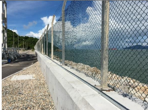
Cooling Water Intake for CCGT Unit No.1
